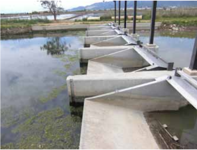
Figure 3: Sluices that allow fresh water to flow towards the salt water side but prevent salt water to flow towards the fresh water side.
