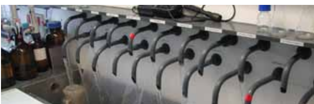
Sampling taps for water quality measurements. An impressive number of 450 compounds is analysed day and night every 1 to 2 hours.
