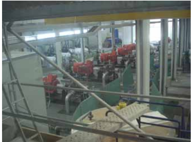
Pumps (red) in the foreground and cartridge filters (white) in the background
