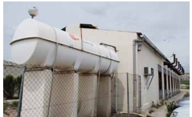
Diesel powered electricity generation unit
