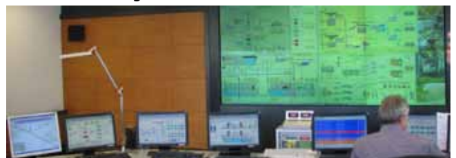
Operator room at the Sant Joan Despí drinking water treatment plant
