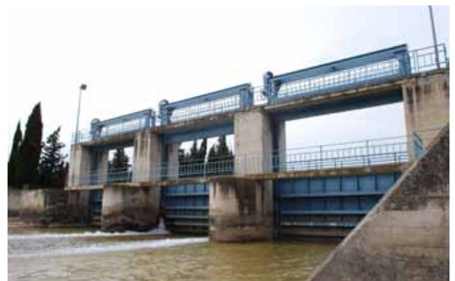
Control sluice at the junction of two main irrigation canals
